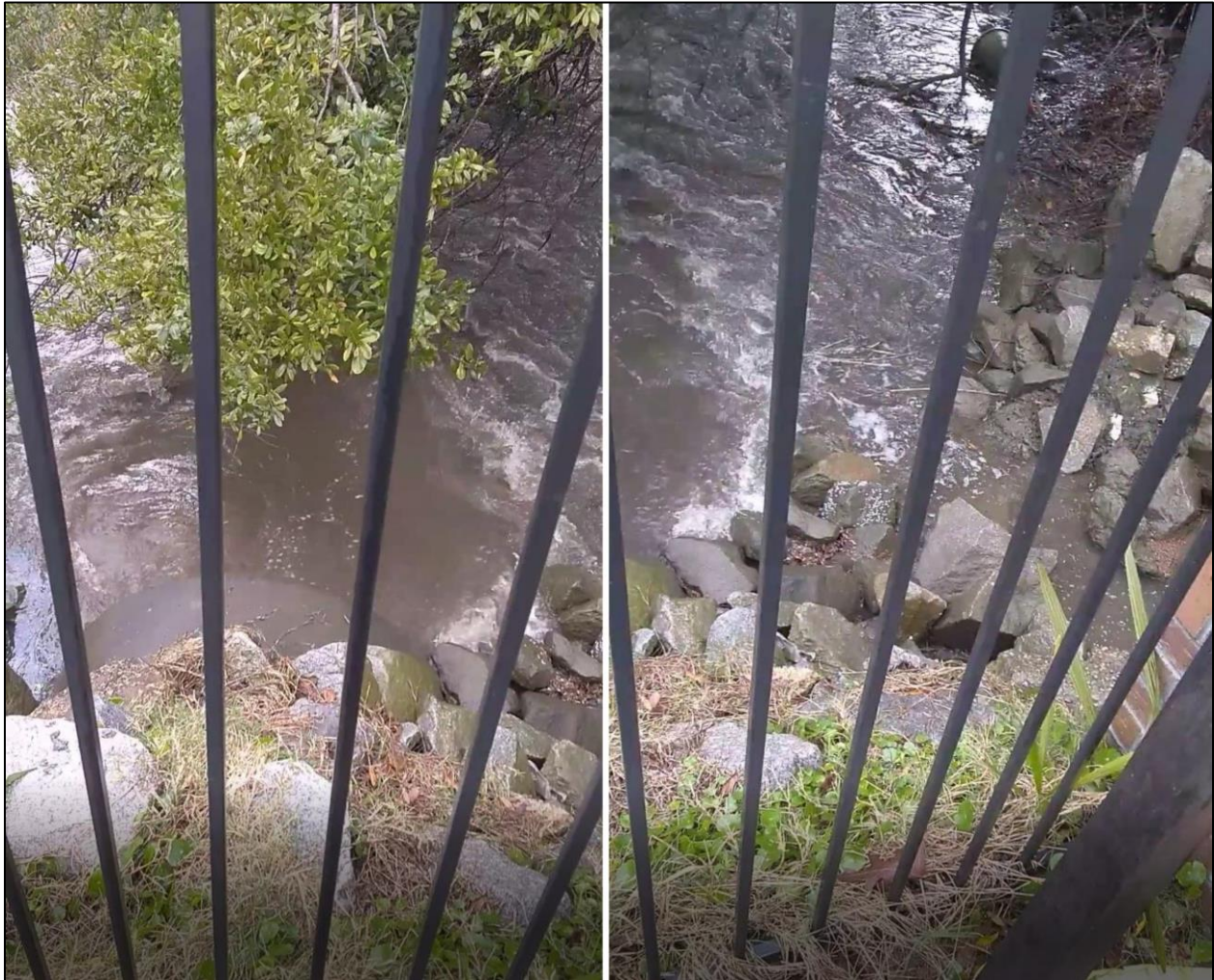
Figure 1. On March 18, 2021, Jimmy Mazyck documented the 48” stormwater pipe at EME Apartments flowing completely full (see left-hand photo). The parallel 42” stormwater pipe was not flowing since it had been sealed with rocks for an unknown reason (see right-hand photo). The location of the pipes is the center of the green circle in Fig. 2. The left-hand and right-hand photos are stills of a video taken by Jimmy Mazyck at 0:39 and 0:28, respectively.
